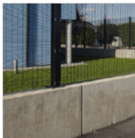
Welded wire fabric fence with board form concrete base
